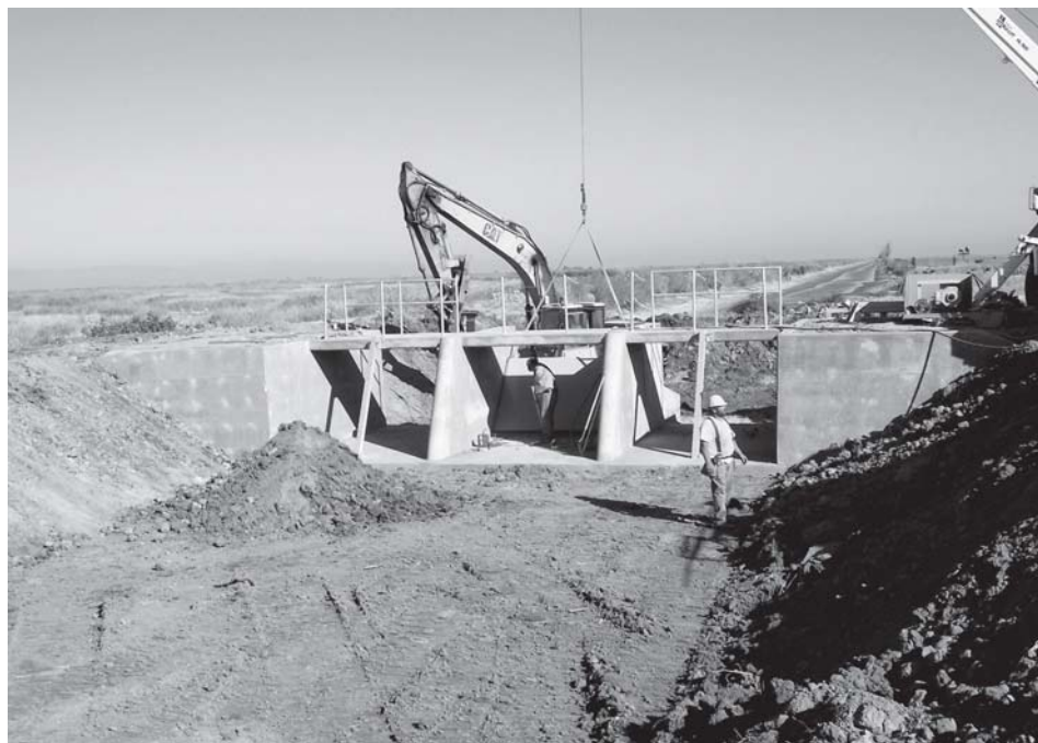
Project Underway — Major work on the Santa Fe Canal will improve water flows to critical wetlands.
